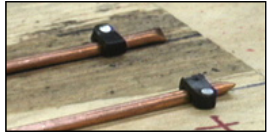
Copper tubing attached to wood.
