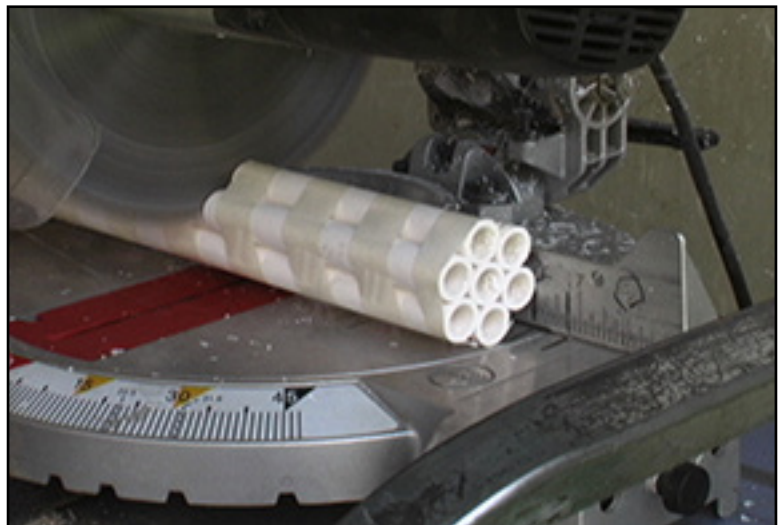
Wrap PVC pipes in bundles of 7 and slice them with a chop saw.
